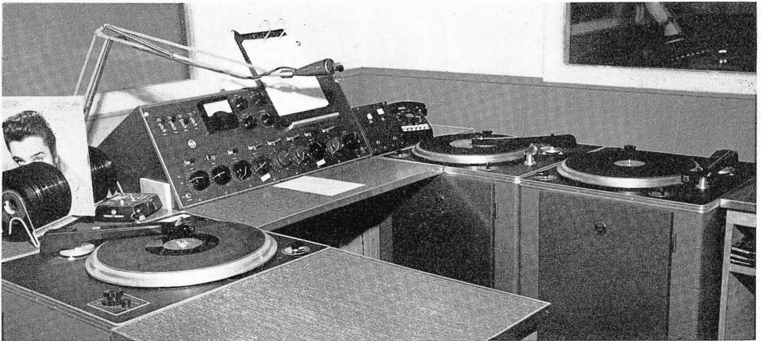
FIG. 3. Typical installation of several BQ-2C's gives a custom look to the studio.
